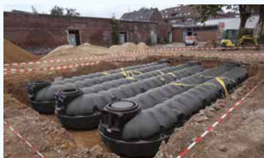
Installation NEO buffertank 3 x 20 000 l
